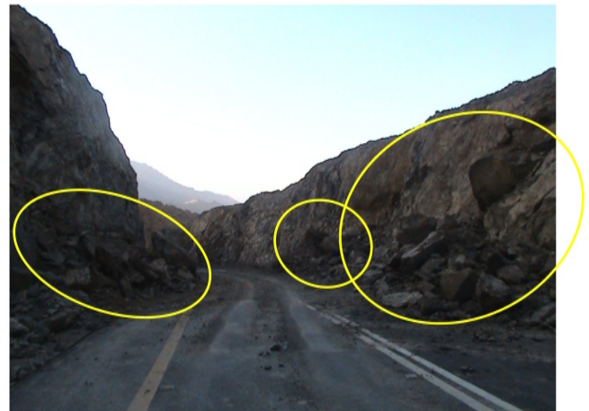
Fig. (4). Rock slope failures shown at yellow circles at the northeast (right) and southwest (left) slope face cuts. Rock blocks were removed aside after the rainfall to clear the road.
