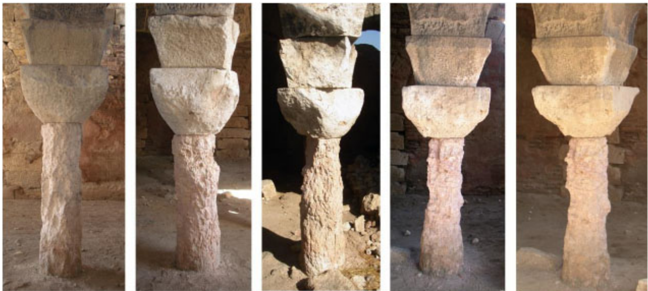
Fig. (5). Decayed columns of the cistern (Column 1, Column 2, Column 4, Column 7, Column 8).
