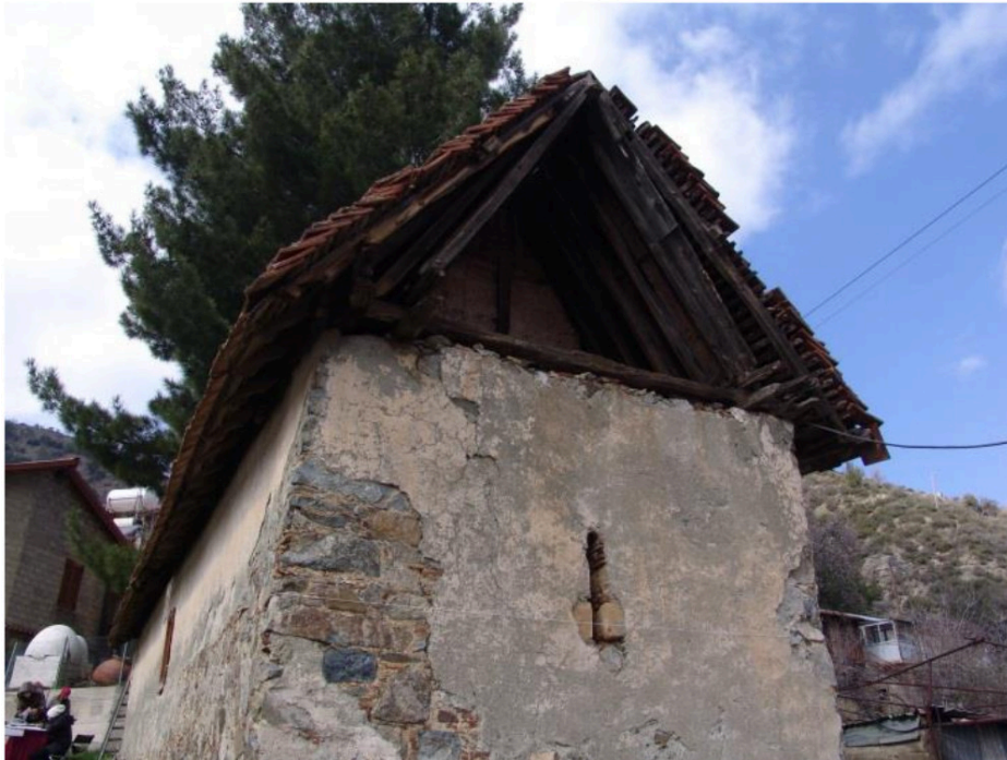
Fig. (1). The single-aisled basilica of Saints Sergios and Vachos, at Kalopanayiotis village. East façade (Photo M.Pelekanos) [4].
