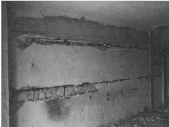
Photo (1). Horizontal cracking due to out of plane shaking of infill walls (Central Greece Earthquake, 1981) Carydis et al. [27].
