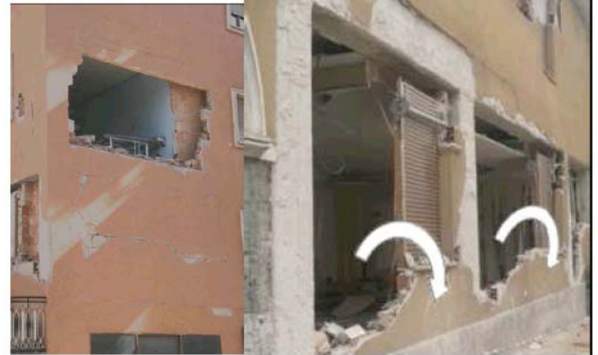
Photo (3). Out-of-plane collapse of infill walls (Abruzzo Earthquake 2009, Vicente et al. [28]).
