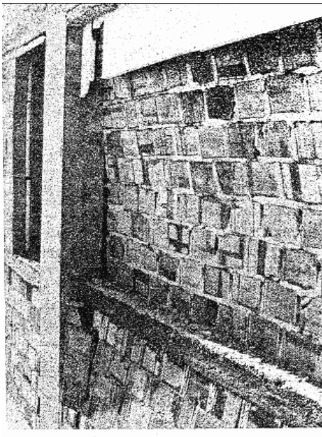
Photo (2). External wall collapse due to out of plane seismic excitation (Kalamata Earthquake, 1986).
