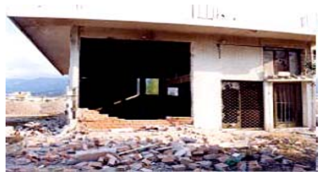
Photo (4). External wall collapse due to out of plane seismic excitation (Athens Earthquake,1999).
