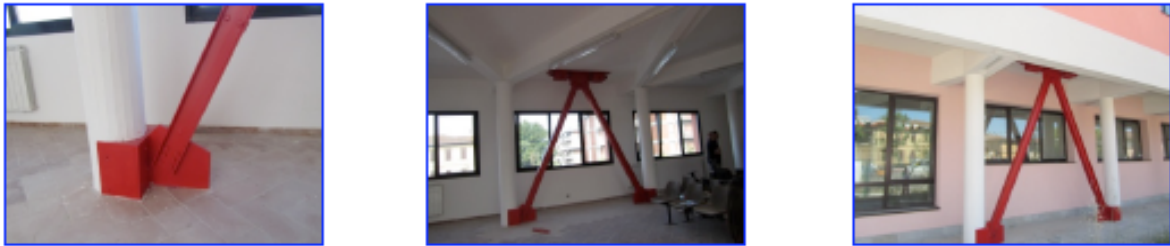
Fig. (17). Detail and general views of the other DB alignment parallel to x in the pilotis wing.
