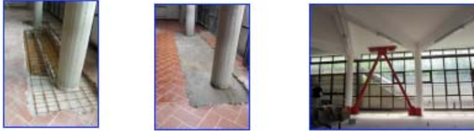
Fig. (16). Construction of the additional R/C beam in one of the two DB alignments parallel to x in the pilotis wing.
