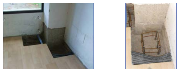
Fig. (15). Preparation of the anchorage zones of braces to the foot of a column.
