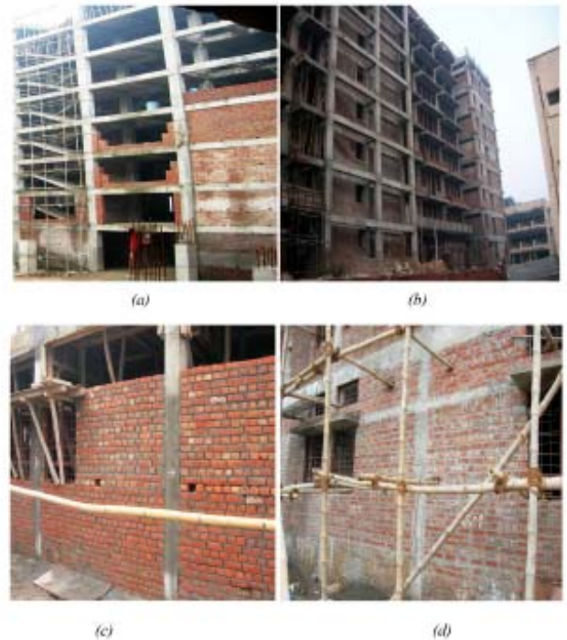
Fig. (1). Photographs showing typical construction sequence of infilled frame building (c) and (d) show construction of lintel band to prevent out-of-plane failure of infills.
