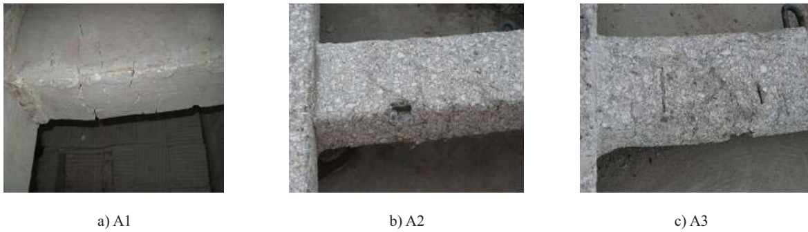
Fig. (5). Cantilever beam after fire.
