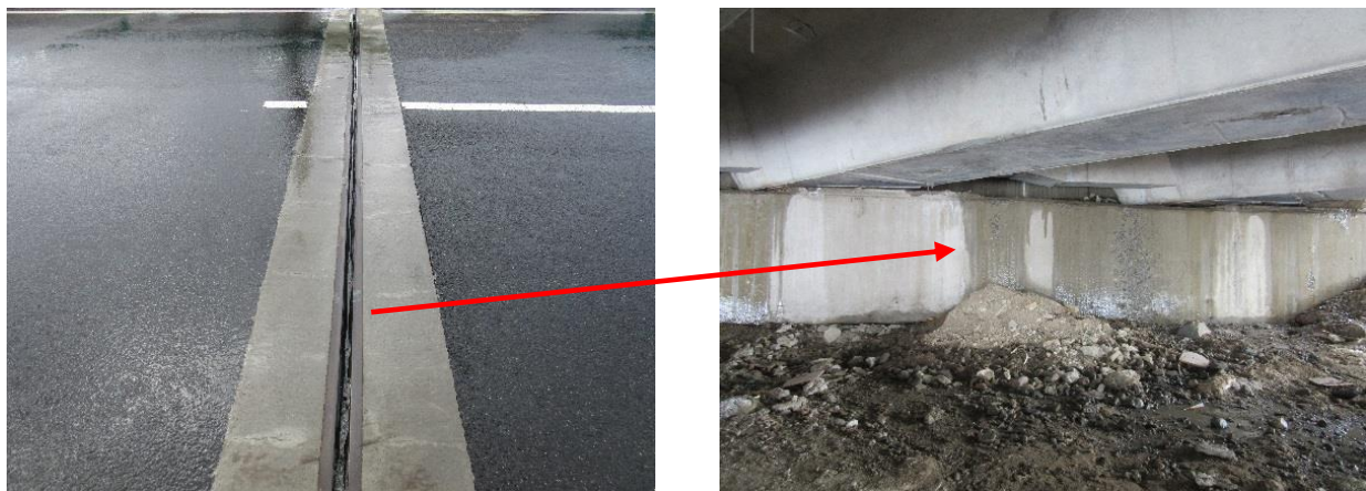
Fig. (9). Breakage of deck joint sealing strip.
