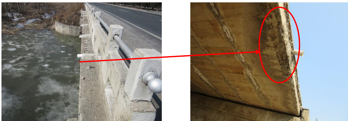
Fig. (11). Short drainage pipes fail and reinforcement corrosion of the side RC hollow-core slabs.
