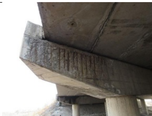
Fig. (7). Concrete scaling and reinforcement exposing of pier.
