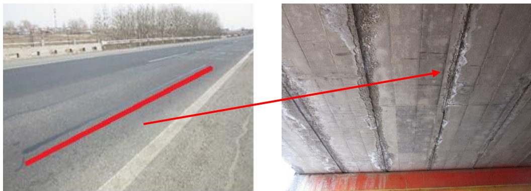
Fig. (8). Longitudinal crack of deck pavement.
