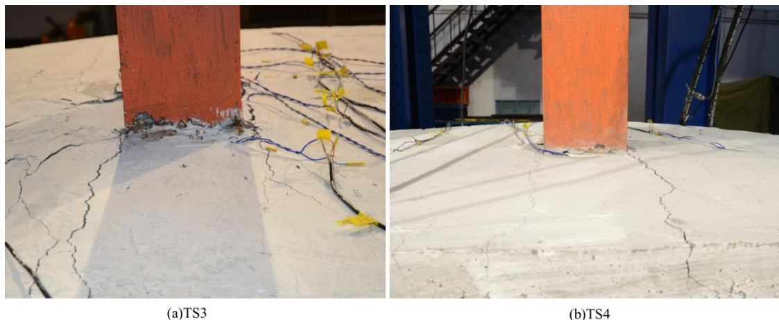
Fig. (13). Failure in test TS3 and TS4.
