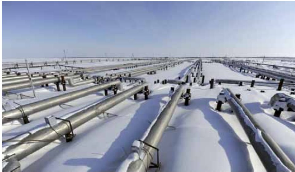
Fig. (4). Inter-connected gas pipelines.
