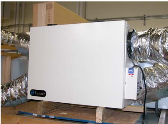
Fig. (2). Ventilation heat recovery (VHR) unit used with the low-cost dehydrator; shown with flexible, insulated duct connections.
