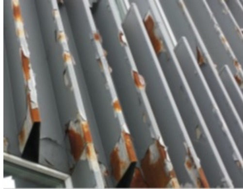
Fig. (5). Corrosion attack on Askja building in September 2013.
