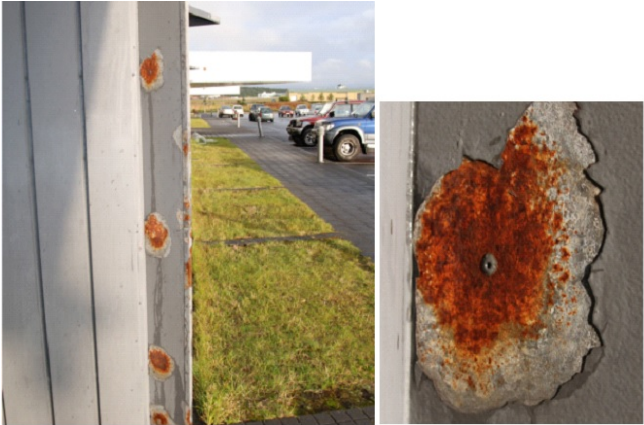
Fig. (3). The corrosion attack related to the stainless steel fasteners. Photos from September 2009 [4].
